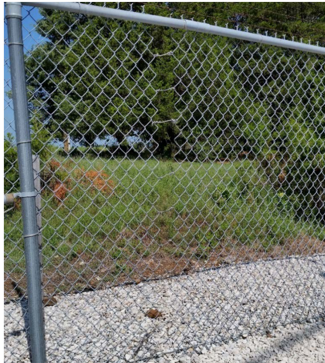
Poor fence repair at the site of a previous break-in compromises security at a tap station and makes it easier to gain access to the asset.
