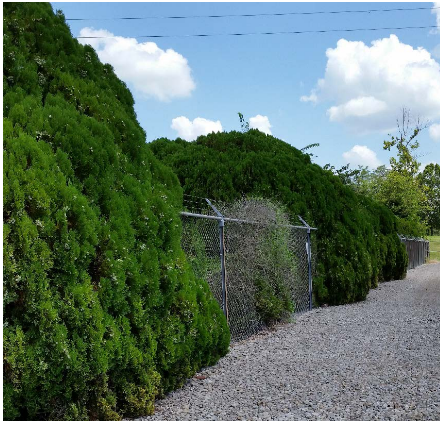
Bushes growing through a fence at a substation create a fire hazard, provide cover to potential intruders, and impair the vision of anyone monitoring the substation.
