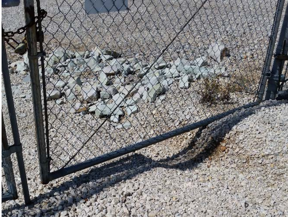
A gap under the fence at a tap station could allow access by a person or animals.
