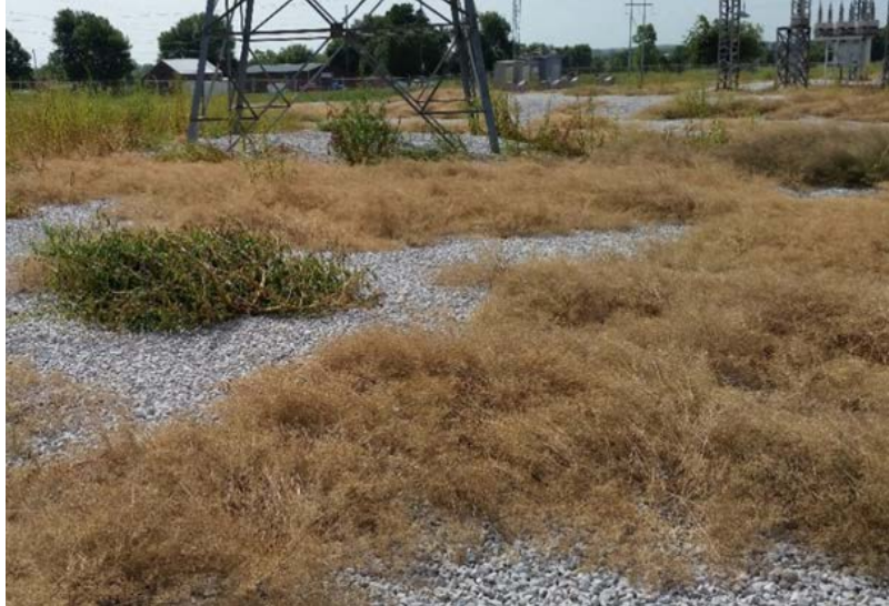
Overgrown vegetation poses potential fire hazard and limits visibility at a substation.
