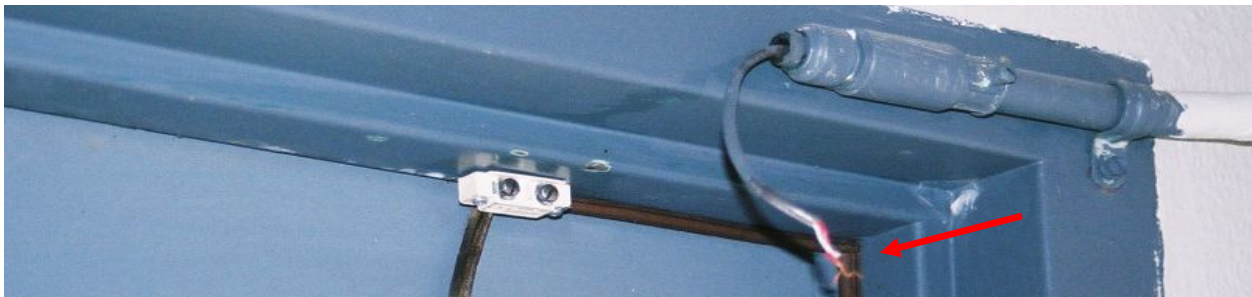
Switching Station Door Alarm Contact – 2004 Assessment Image
