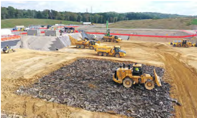
At the OSWDF, placement operations continue as a landfill compactor compresses debris from the X-326 demolition project.
