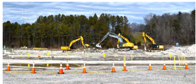
Heavy equipment tears up the largest remaining slab at ETPP, which was where the former Centrifuge Complex once stood.
