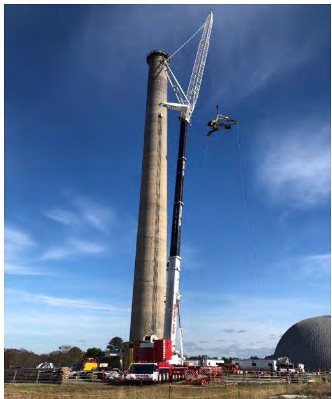
A patented concrete chimney demolition system called the MANTIS is being lifted by crews to the top of the exhaust stack.
