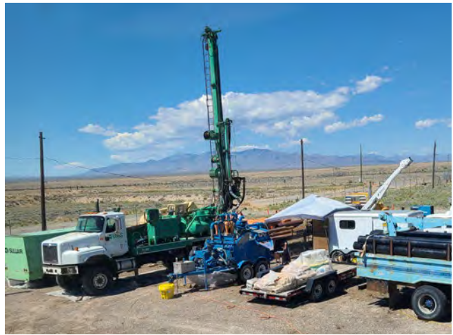
Crews drill a new well near Test Area North at the INL Site.
