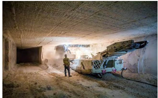
A continuous miner machine in WIPP's underground chews through a final section of salt to finish the preliminary rough cut of Panel 8.
