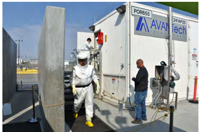
Following installation near the AP Tank Farm and rigorous testing, the TSCR is ready to start treating tank waste in 2022 to build up a large supply of liquids that can be fed directly to the nearby vitrification facility beginning in 2023.
