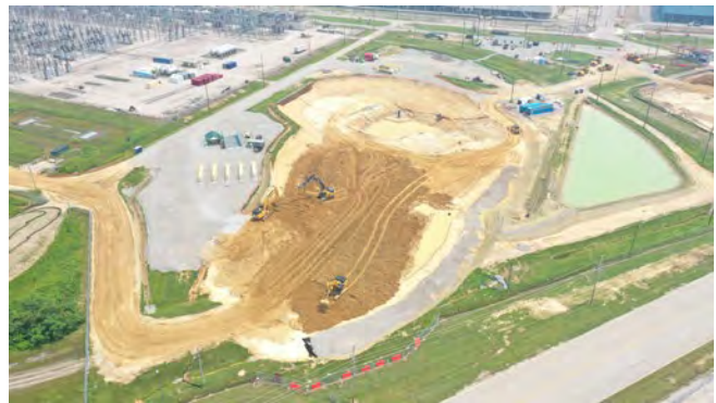
A northeast aerial view of the X-740 Groundwater Plume Excavation Project shows continuing progress on the site's west side.
