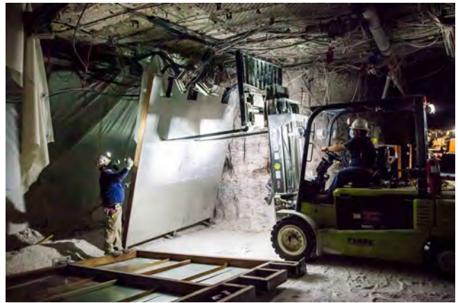
Workers in the WIPP underground install a bulkhead as part of a two-month maintenance outage.
