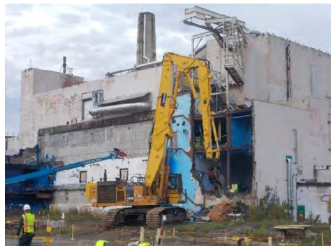
A large excavator is used to remove the west wall for continued deactivation work inside the Acid Recovery Cell.
