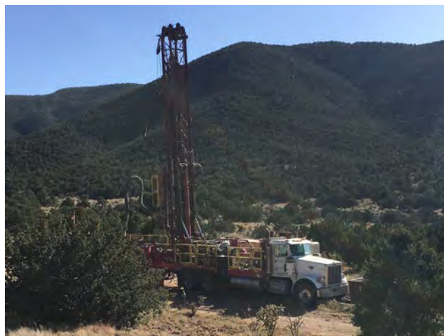
Installation of a groundwater monitoring well at the Burn Site Groundwater AOC.
