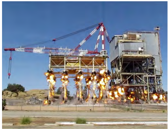
ETEC's final building for demolition – the Sodium Pump Test Facility – amid blasts from shaped charges.
