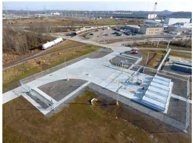
Aerial view of the bulk hydrogen system at the Portsmouth DUF6 facility.
