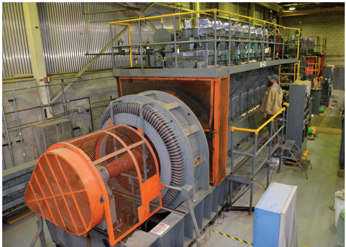
IRA-funded ATR enterprise backup-generator replacement
