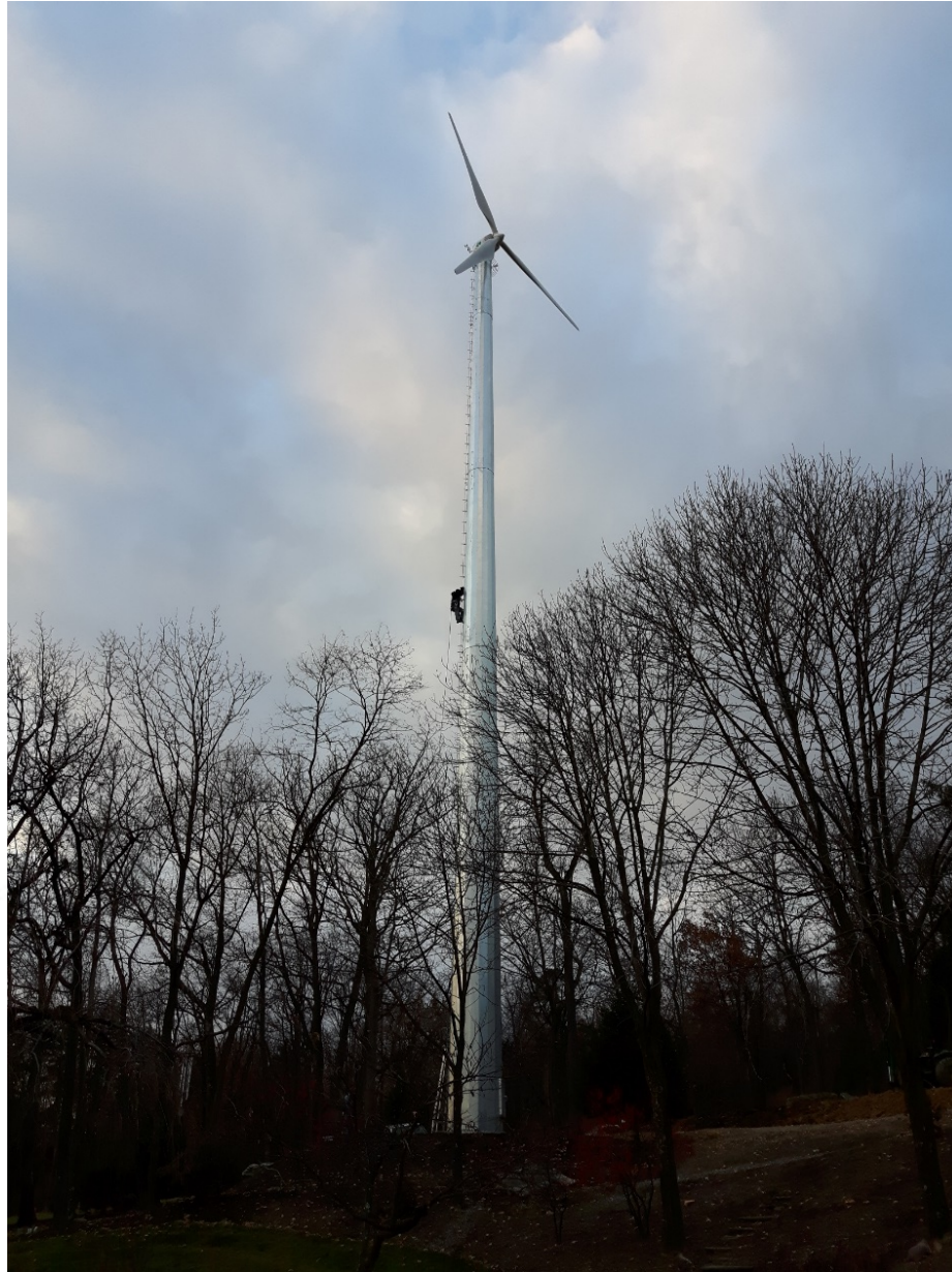
Installer Roger Dixon of Skyland Renewables climbs the Eocycle tower during turbine construction at a York, Pennsylvania residence. Photo courtesy of Eocycle
